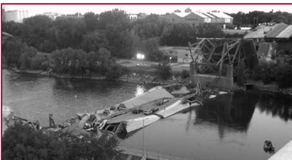
The I-35W bridge over the Mississippi River collapsed August 1.
